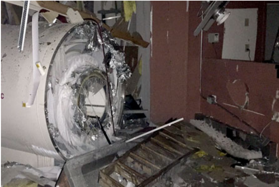
MR scanner explosion
