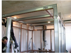
the basis of the magnetic shielded room is an aluminium frame
